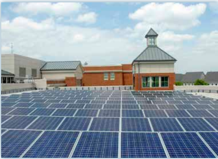
Solar photovoltaic panels installed on the roof of Lakelands Park Middle School.
