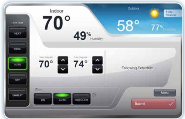
WiFi-capable thermostats will be installed in relocatable classrooms in Summer 2018.
